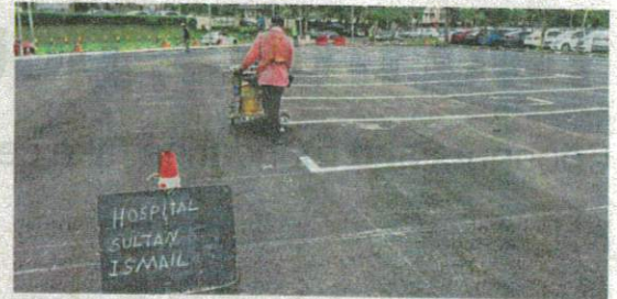
Less worries: An additional 88 parking bays will be added at Hospital Sultan Ismail to overcome the congestion problem.
